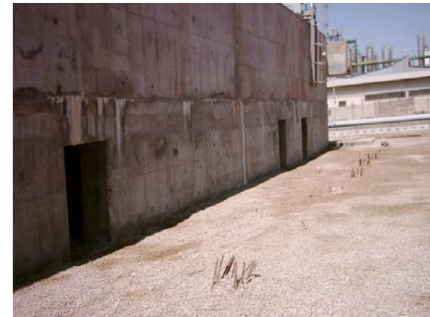
Leakage at NPC
